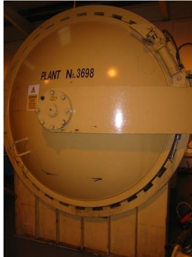
Autoclave in position
